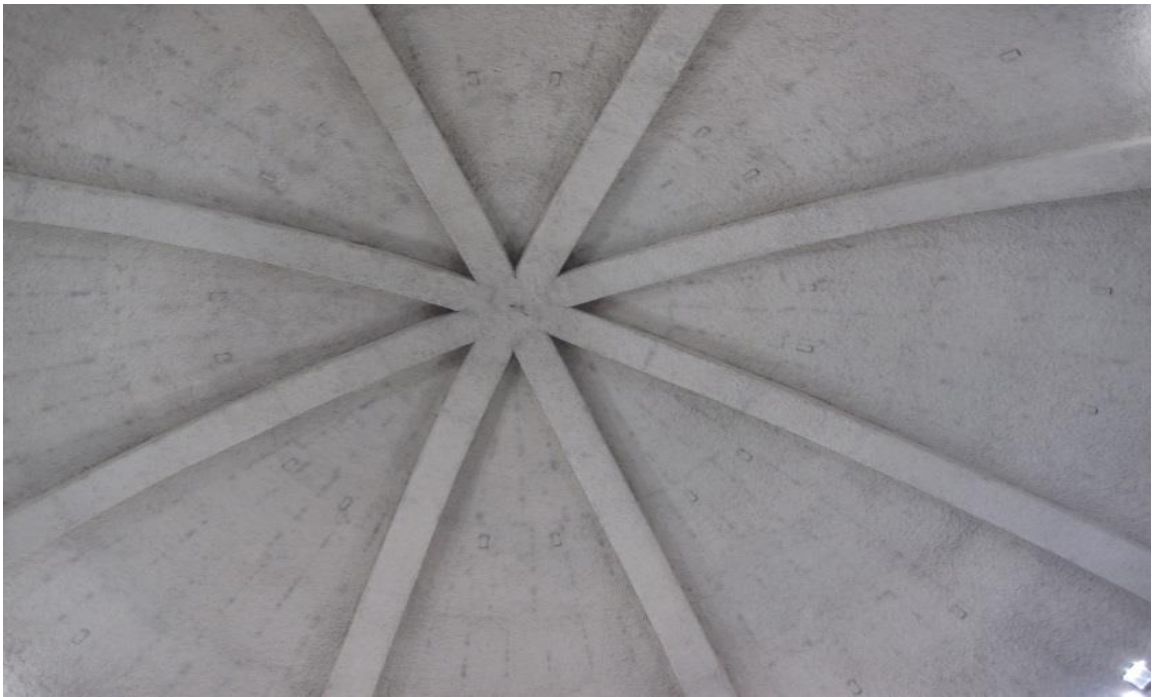
Figure 5-Use of polyurethane foam as fire resistant on steel structure dome; in the New Afghanistan Parliament Complex - Kabul
